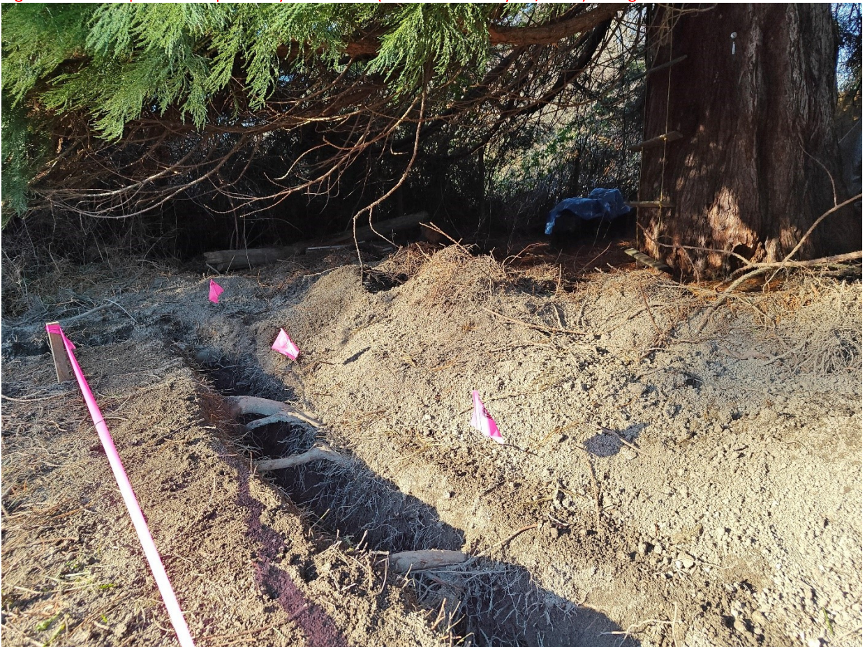
Figure 12. View of west side of exploratory trench and root locations 9, 8, and 7 (from left to right).
