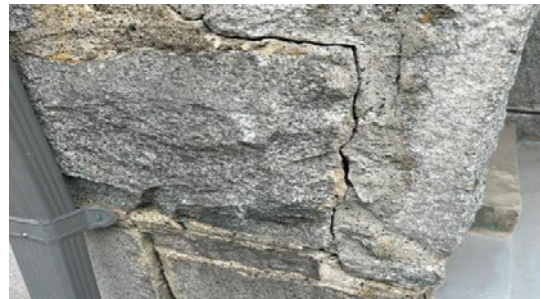
crack in foundation to be repaired in 2025
