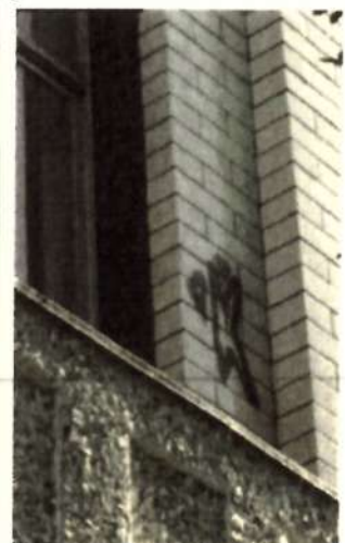
Graffiti on glazed brick.
