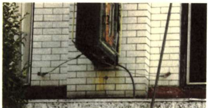
Staining on glazed brick below blade sign.
