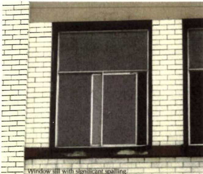
Window sill with significant spalling.
