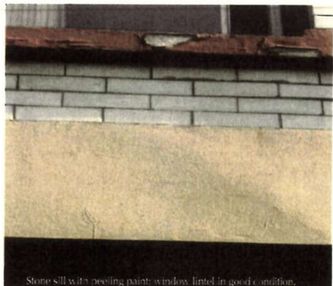
Stone sill with peeling paint; window lintel in good condition.
