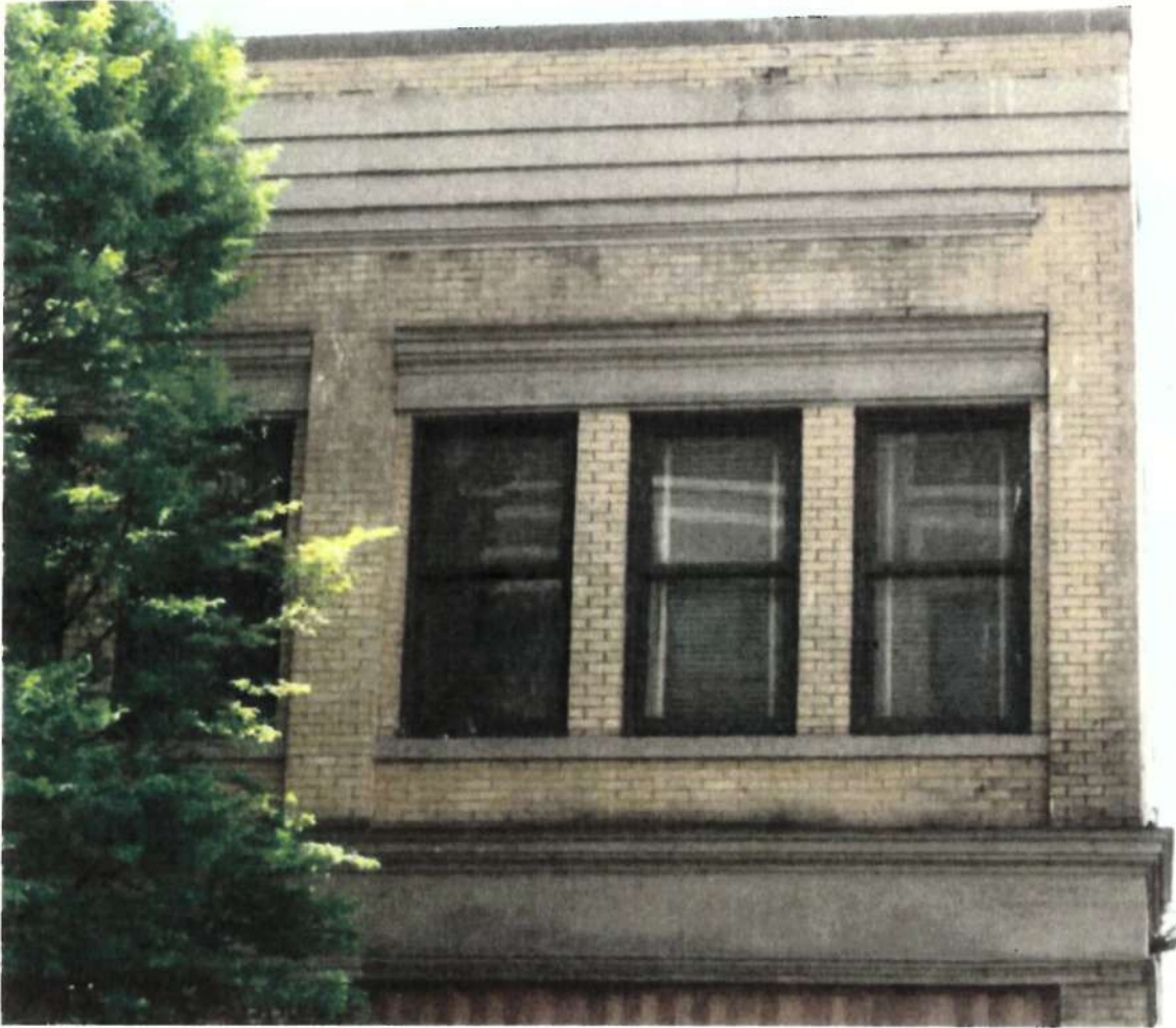
Photo showing partial exterior masonry wall above the storefront. Note typical deterioration of masonry wall.
