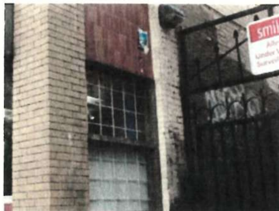
Photo showing storefront return, and partial masonry wall along the laneway elevation to the east; note tilework at the storefront transom that are not original and should be removed.
