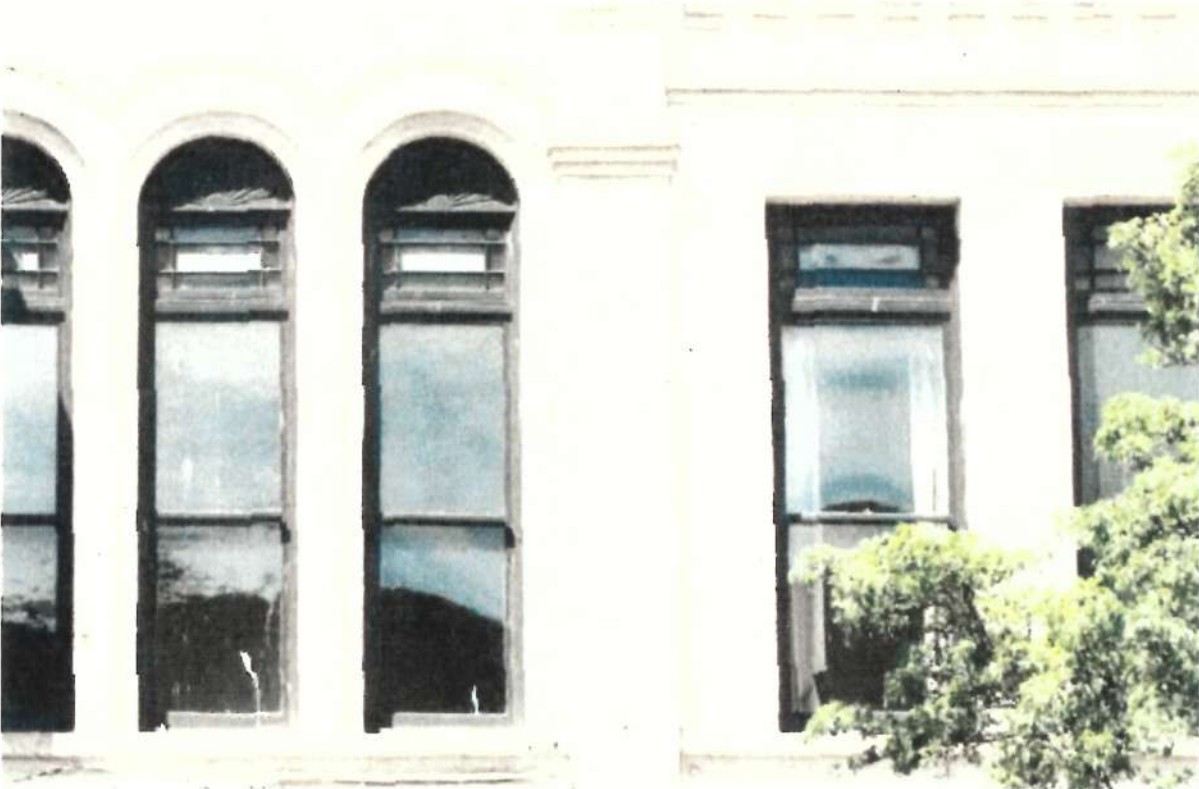
Detail photo partially showing existing window openings, with surviving original wood window assemblies at the upper level of the historic street facade.
