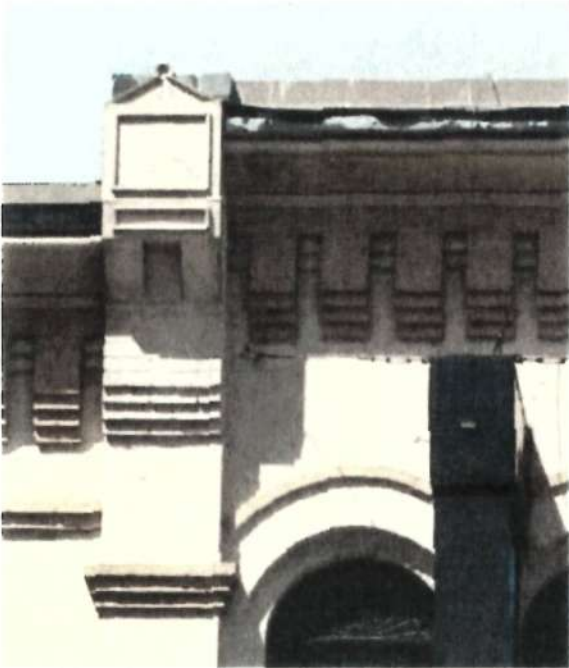
Detail photo showing typical condition of architectural brickwork detailing and metalwork along parapet level.
