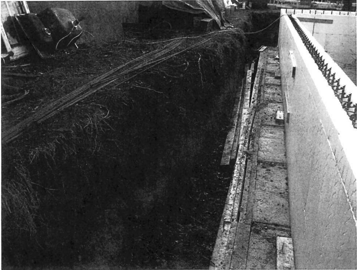
Picture 1: View of edge of excavation showing no large roots exposed (picture supplied by client).
