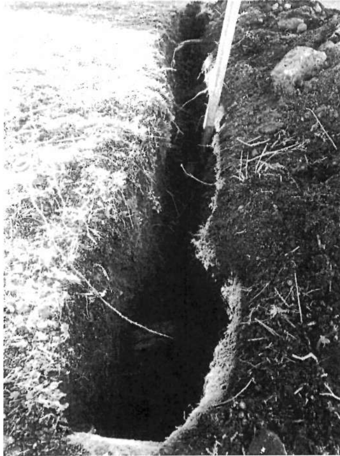
Photo 2: 7cm diameter retained root in foreground near existing retaining wall.
