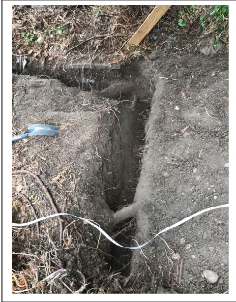
Roots encountered at north east corner
