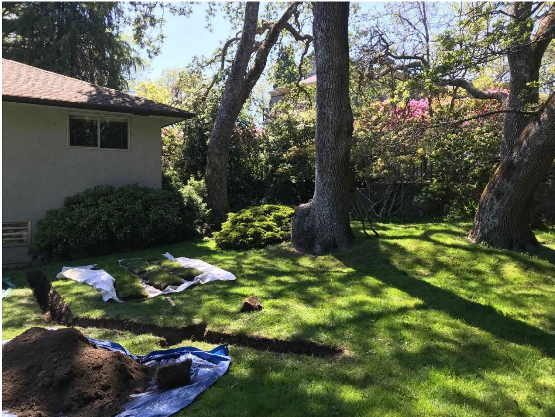
A trench was hand-dug at the approximate location of the proposed foundation excavation, 4.5m from Oak #201.
