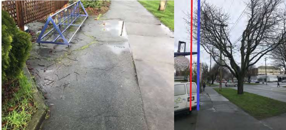
Picture #1 (left) showing the cracks likely caused by roots of Horse Chestnut #2. All roots within private property will be removed due to the underground parkade excavation to the property line (the edge of the concrete sidewalk at the top and bottom of the photo).
