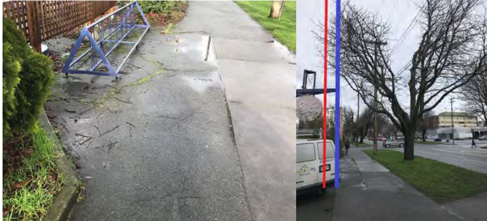
Picture #1 (left) showing the cracks likely caused by roots of Horse Chestnut #2. All roots within private property will be removed due to the underground parkade excavation to the property line (the edge of the concrete sidewalk at the top and bottom of the photo).
