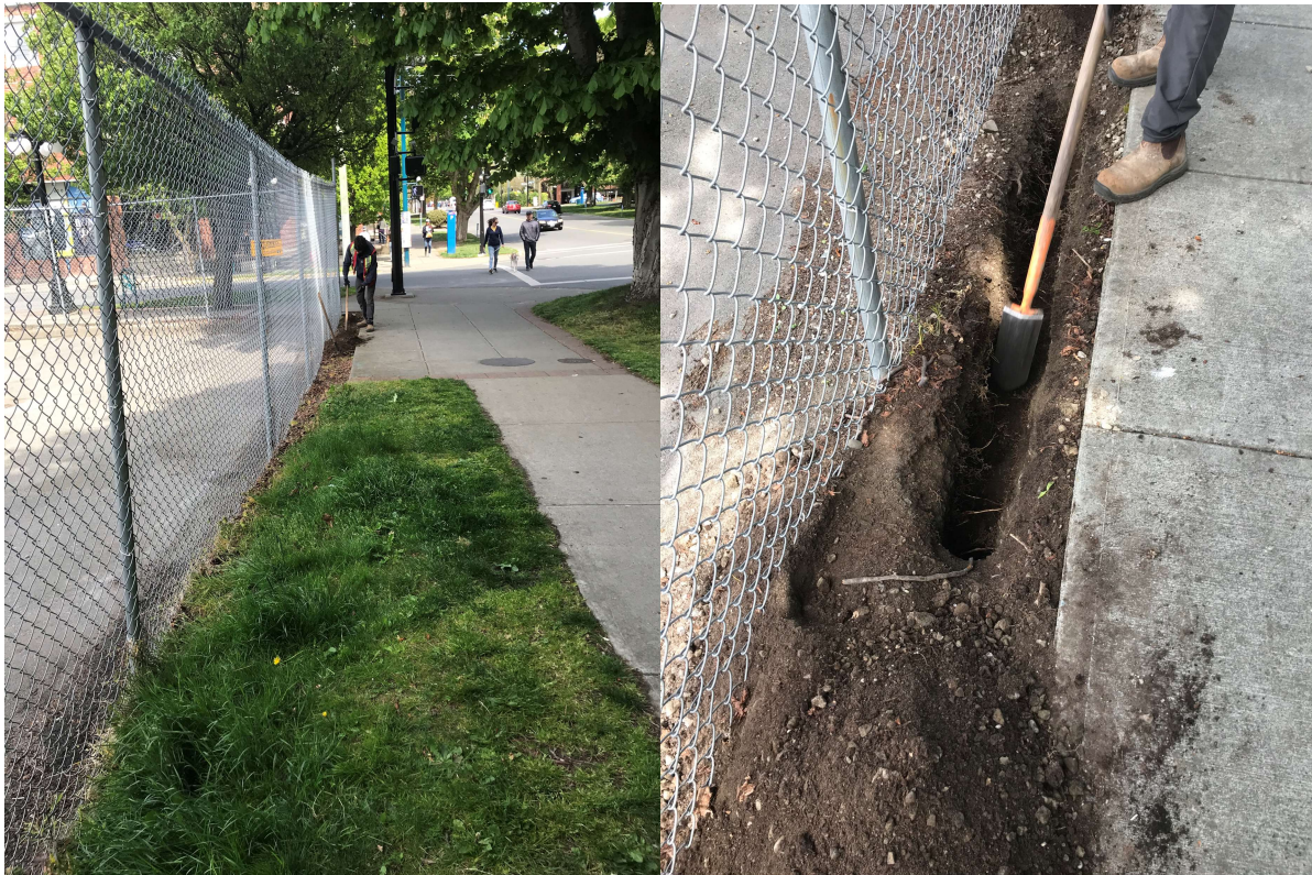
Locations of exploratory excavations on Vancouver Street frontage. Depth of excavation limited by underground concrete structure.
