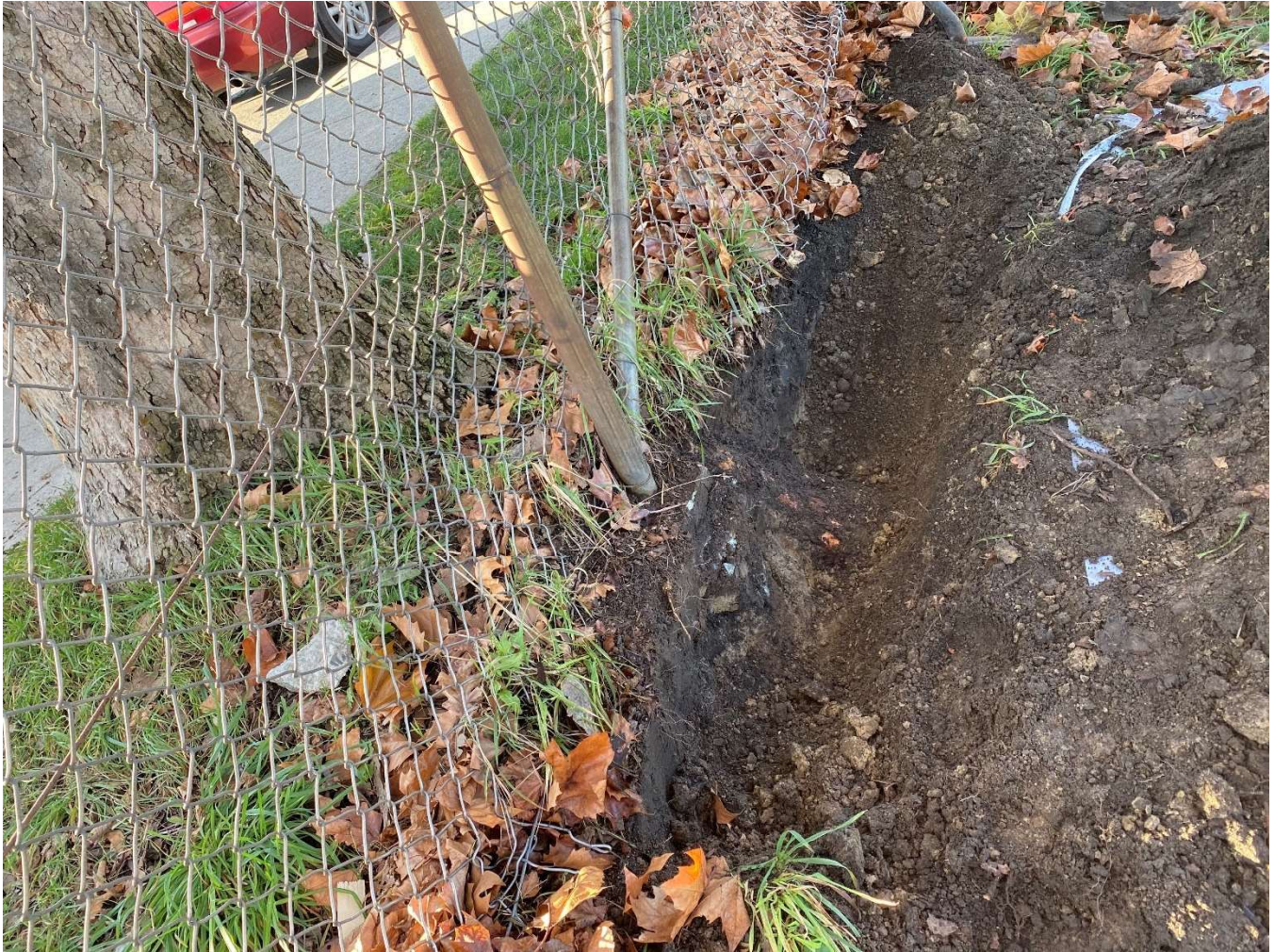
Photograph 4 – Municipal London Plane (NT5) – Exploratory excavation to determine root depth within the proposed sidewalk footprint.
