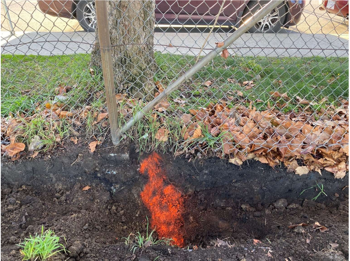
Photograph 5 – Large buttress root (painted orange) found within the exploratory trench. No other roots were found during exploratory excavation.
