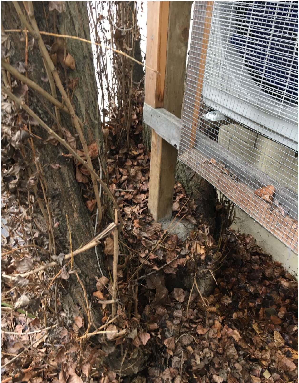
Figure 10. Trunk of tree 155. Multiple codominant stems with epicormic growth. Cement footing poured in trunk cavity.
