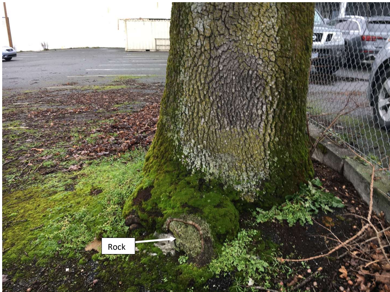
Figure 7. Trunk and root crown of Tree 151. Note rock enveloped by tree. Rooting area is restricted by pavement.
