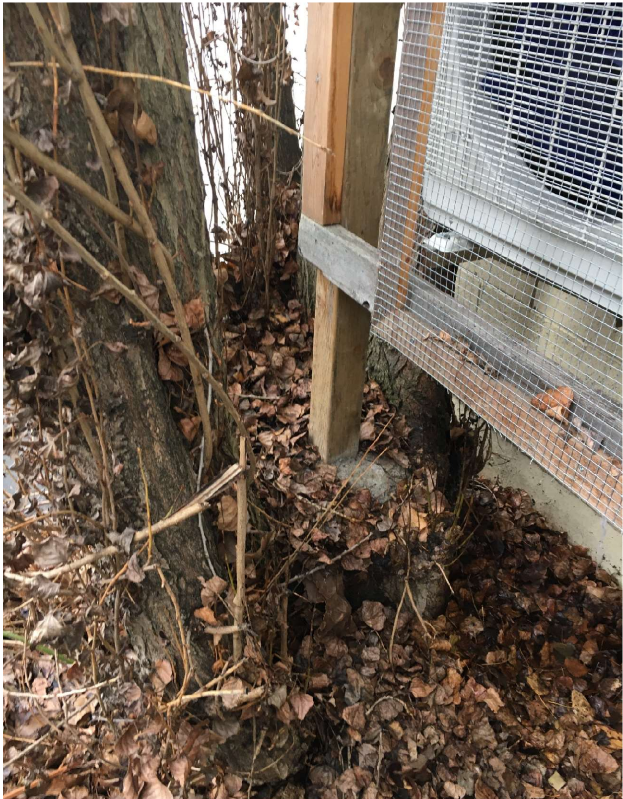
Figure 10. Trunk of tree 155. Multiple codominant stems with epicormic growth. Cement footing poured in trunk cavity.
