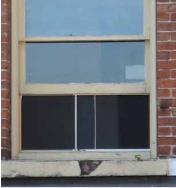
Above: Parge brick sill of rear façade window showing deteriorated parging.
