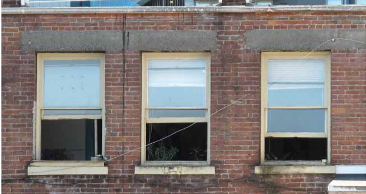
Above: 1-over-1 hung wood sash and frame windows on rear of building. Most windows appear to still have an operable lower-sash, unknown if upper-sash can be lowered. Concrete lintels span one to two window openings. Deterioration evident on sills lower jambs, bottom rail. Localized areas of paint failure present. Staining on and around brick sills.
