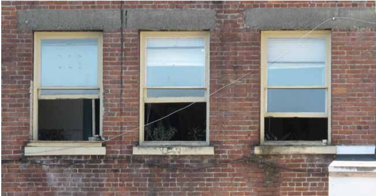
Above: Typical deterioration of masonry on rear of building including staining, cracked bricks, mortar loss, efflorescence and past unsympathetic repairs.
