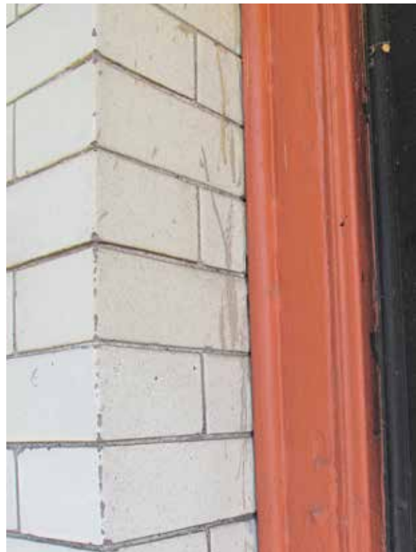
Above: Typical brick damage of chips and paint on brick face from painting adjacent wood elements, present on both "street" façades.
