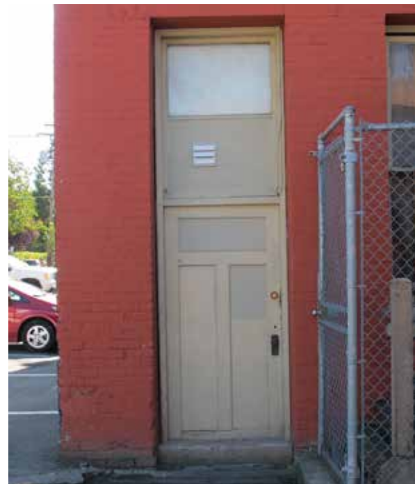
Below: Wood door, frame, and transom on rear façade ground floor intact. Transom glass removed and/or boarded over. Brass hardware of door intact. Lower extent of door and sill shows signs of deterioration.
