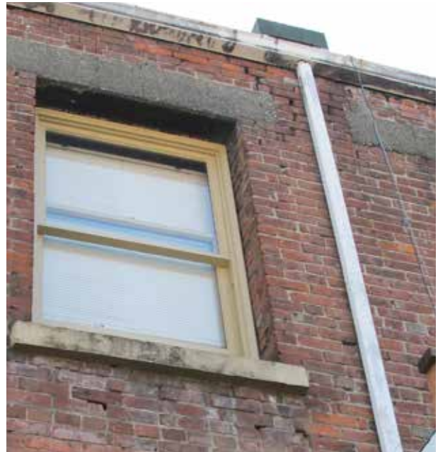
Above: Mortar loss, distortion of brick, and staining on rear of building likely caused by overflowing gutters and undersized downspout.
