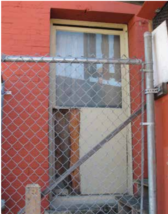
Below: Window on ground floor of rear façade with missing glass and loose upper sash.
