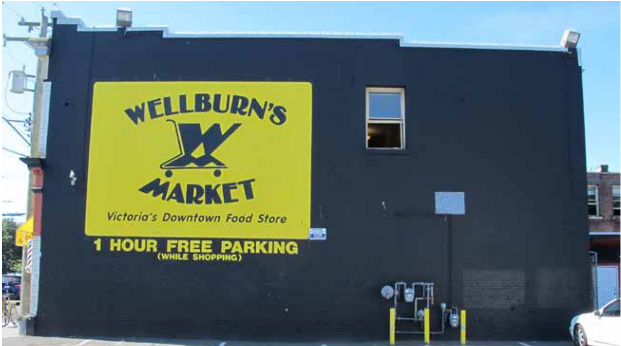
Above: Painted brick of the north façade. Paint is a later intervention and limits assessment of underlying brick. Surface damage to some brick and mortar loss present in areas at base of wall at approximate height of car mufflers and bumpers.
