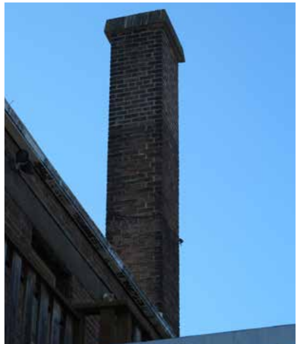
Above: Brick chimney with concrete cap. With proposed demolition of building, chimney brick could be salvaged for reuse.
