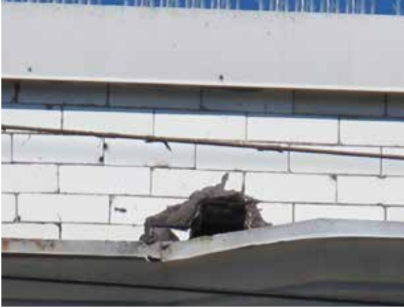
Above: Later installed scupper above roof cornice on Cook Street façade. Weather proofing material applied onto the face of the parapet.
