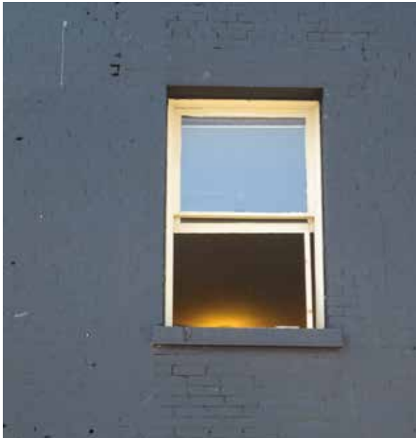
Above: Typical example of mortar loss and unpatched past penetrations in brick wall on “non-street” façade.
