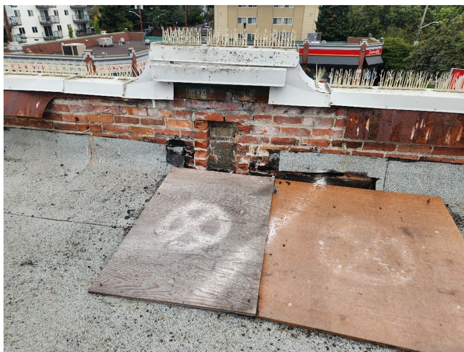
Figure 8 – Deteriorated Roof and Parapet Condition
