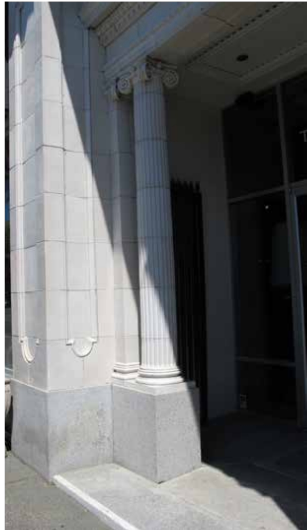
Below: Grey granite base at columns and step of portico. Localized chips and staining on granite.
