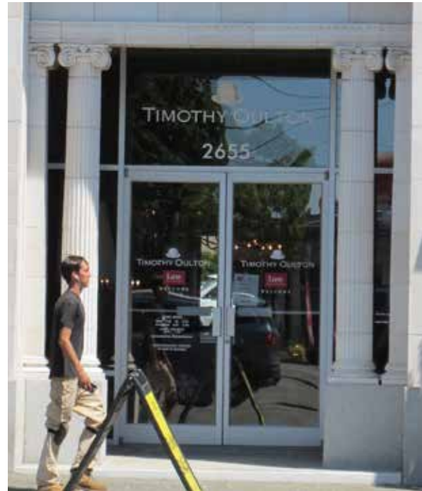
Left: Replacement aluminum door assembly of Douglas Street entry. New wood door assembly should be installed and existing aluminum assembly removed.
