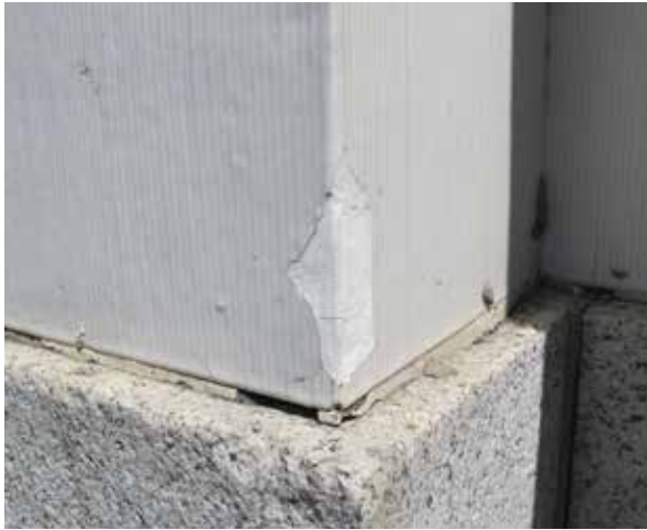
Above: Example of combed finish of terra cotta. Finish has been damaged exposing biscuit underneath. Mortar loss also present throughout.
