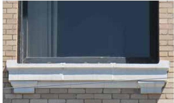
Above: Glazed terra cotta window sill typical of third floor windows on primary façades. Sills in good condition. Some sills appear to have been unsympathetically repointed in the past.
