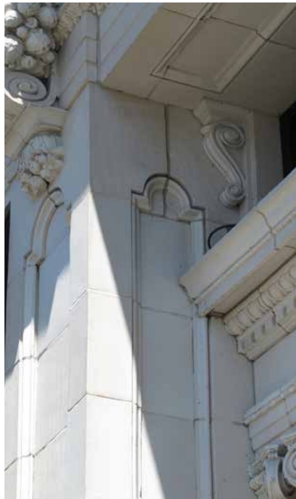
Above: Terra cotta cladding on column at Douglas Street entry. Columns have sunk panels on front and inside faces. Hairline cracks present in some of the terra cotta pieces. Mortar loss and stained mortar joints present.
