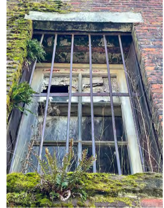
EXISTING WINDOW CONDITION TYP.
