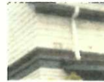
PAINTED COMMON COURSED SAWN CEDAR SHINGLES WITH TAPER. PAINTED EX 6" BEADED SHIPLAP SIDING.
