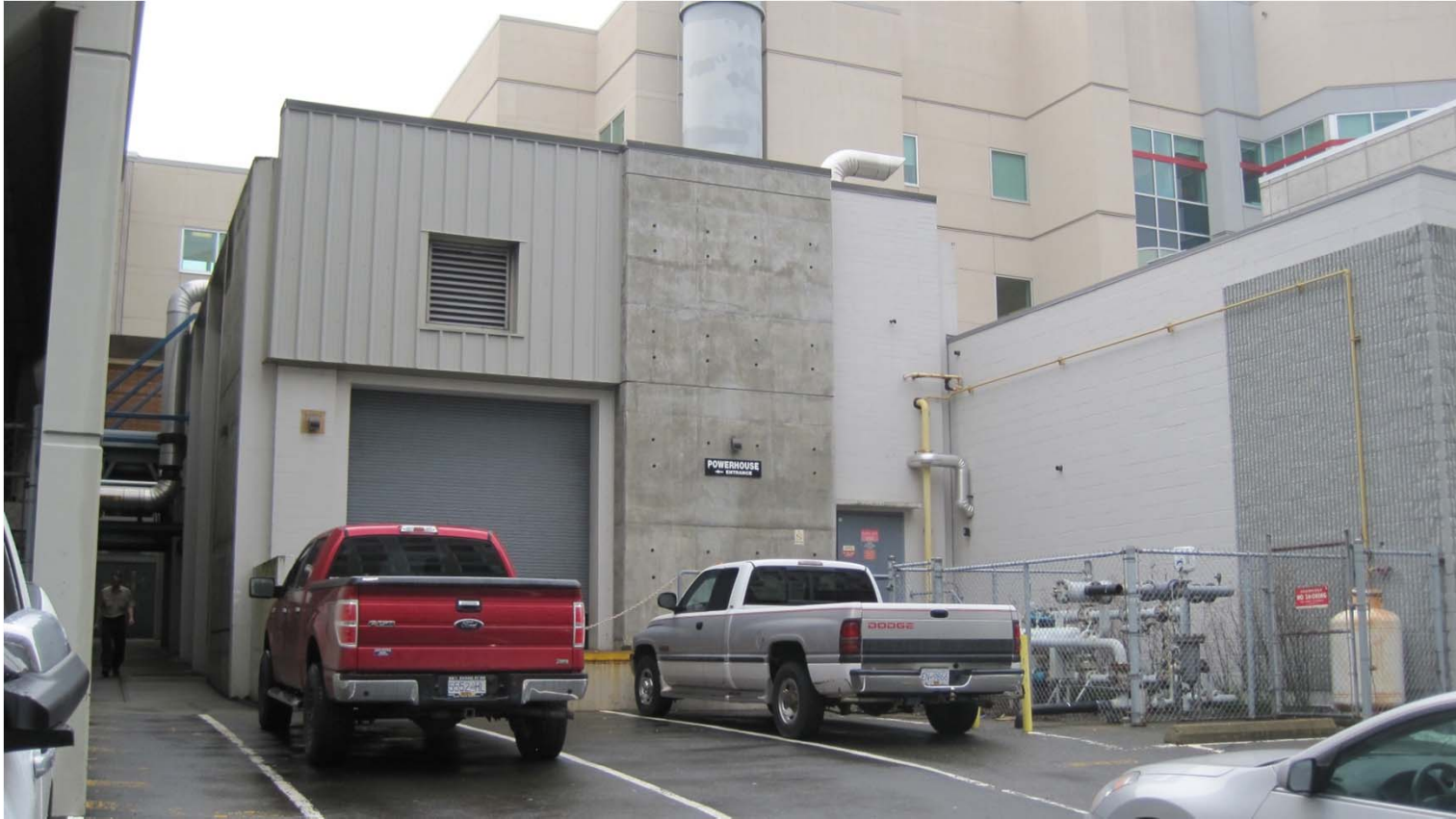
Existing Boiler House
