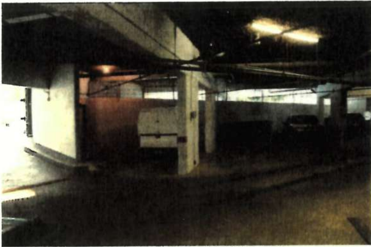
AUG. 01/17 6:30PM LEVEL B-2 (ENTRY GATE)
